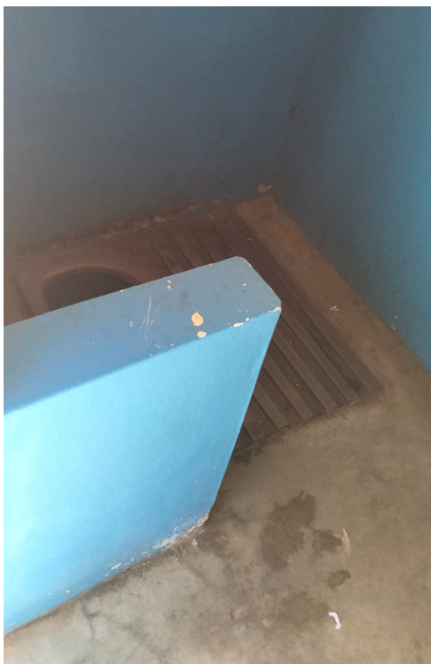
^ this is what the current toilet system looks like at Thusanang
